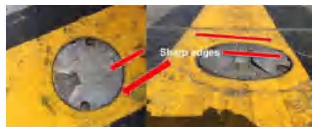
Figure 8. Lights type used in the parking bays - OMAA
